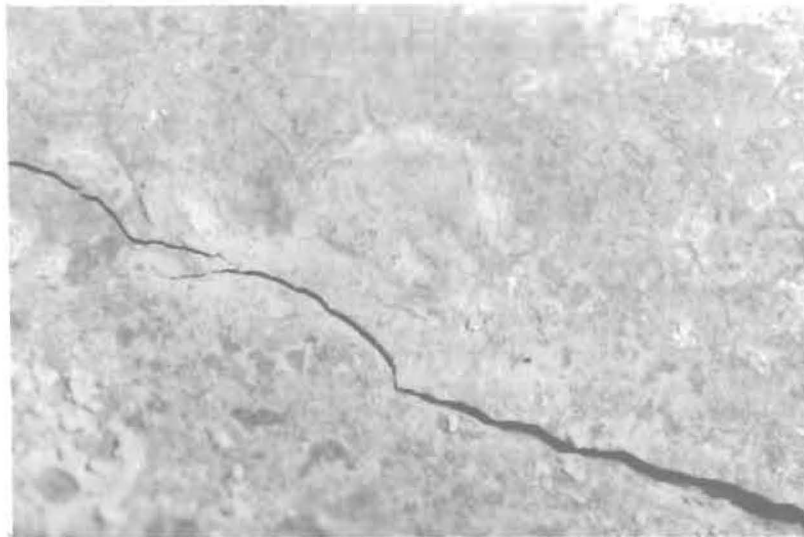
c) THE CRACK PROPAGATION AREA
