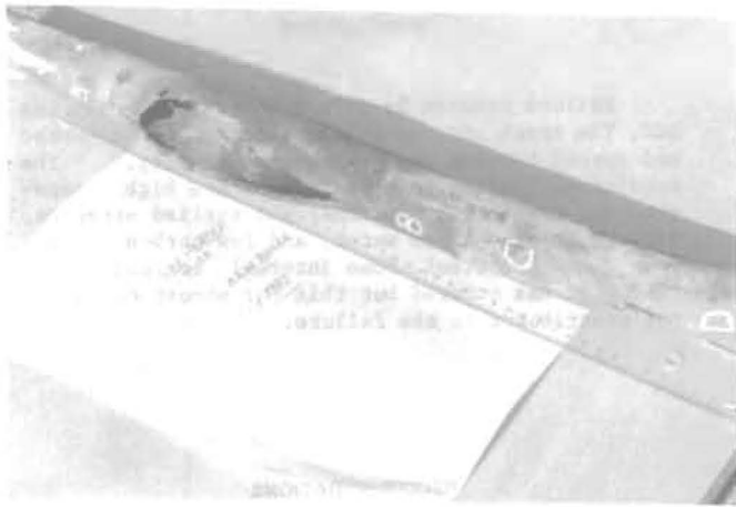
a) THE FAILED TUBE - OVERALL VIEW
